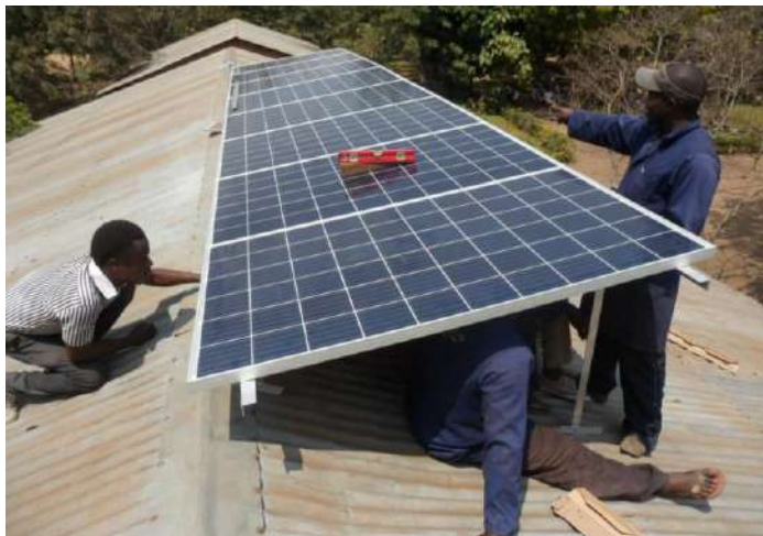
Photo 1: Solar artisans installing a solar system at Igawa Secondary School, Malinyi ©TAREA
