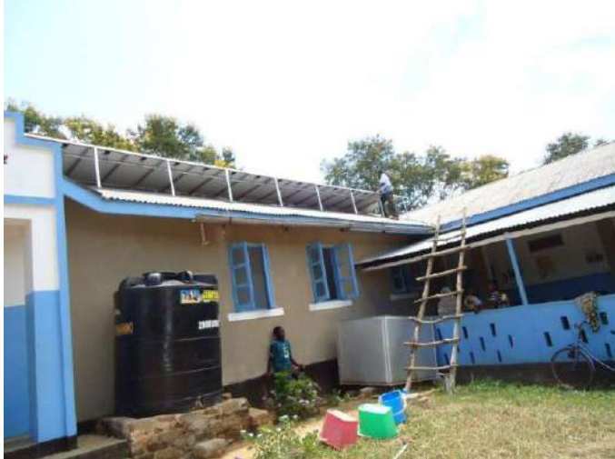
Photo 20: Solar photovoltaic system at Magubike Health Centre, Morogoro Region ©TAREA
